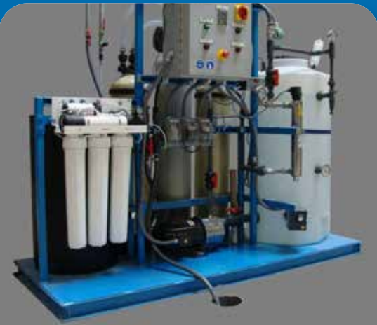
WATER TREATMENT SYSTEMS
