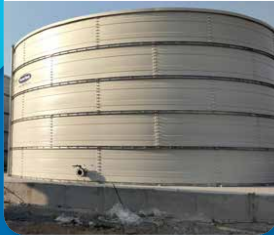
WATER STORAGE TANKS
